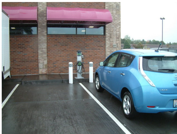
Figure 3.2: Photos of Typical EVSE Stations
